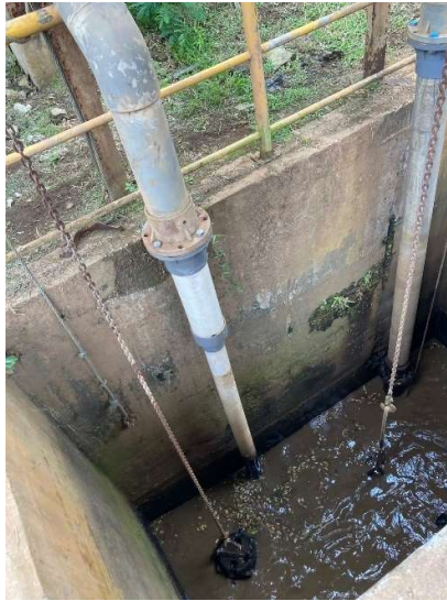
Gambar 4.5 Pompa Sumpit Drainase IPA Cilandak
